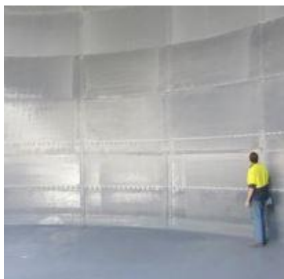
Figure 1. Steel bolted panel tank lined with Tufflon-P90. Used for remote community drinking water supply
