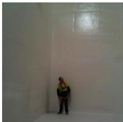
Figure 2. Concrete tank lined with Tufflon-P90. Australia's first water recycling plant producing potable quality water
